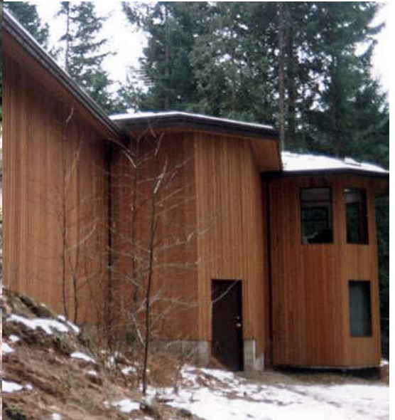
Below: We covered the west wing and basement until we could afford to buy more windows. Climbing to the roof from a ladder to remove the leaves from the gutters was a dangerous semiannual chore.
